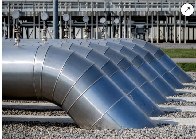
Pipes at one of Europe's largest interconnection gas hubs at Baumgarten an der March, Austria. Photographer: JOE KLAMAR/AFP via Getty Images
